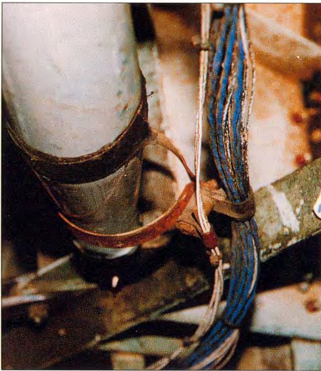
After years in service this clamp has slipped down the tapered strut and the harness is not held securely.
