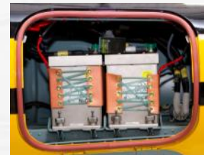
H130 SECONDE BATTERY INSTALLATION
