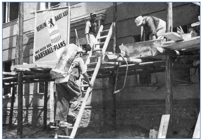
Construction workers in West Berlin, West Germany, work on a project funded by the United States under the Marshall Plan. (National Archives)
