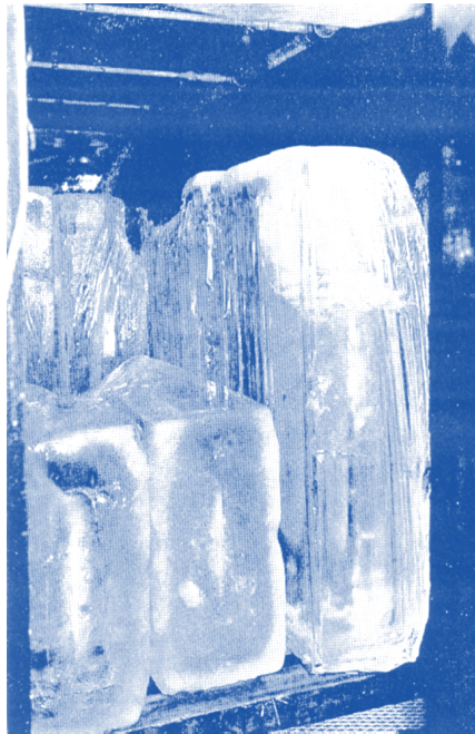
Figure 5: Ice blocks inside air cooler.
