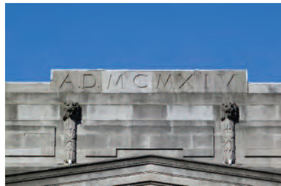
(fig. 127) UNIVERSITY COLLEGE DUBLIN A detail of the grey Stradbally limestone with stylised lion masks on tied reed pedestals. The blocking course, inscribed with the date of construction in Roman numerals, was originally intended to support a pedimented tower, but limited finances precluded its completion.
