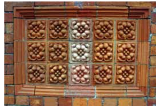
(fig. 119) FAÇADE DETAIL, FORMER CUNARD LINE OFFICE (NOW PERMANENT TSB BANK) West Beach, Cobh (c.1890)
