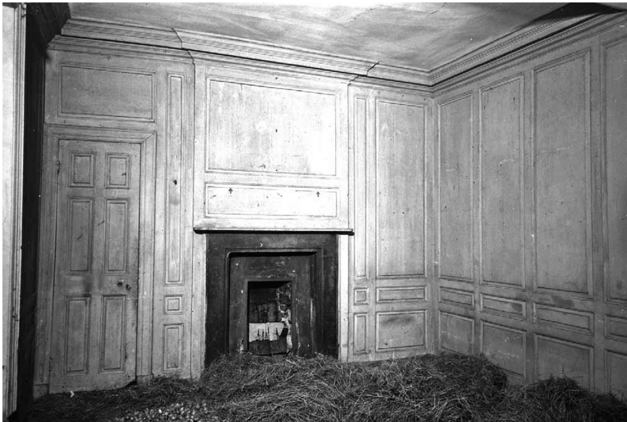
MOSSTOWN HOUSE Mosstown Demesne, near Keenagh (built or rebuilt c. 1660 and altered c. 1730)
