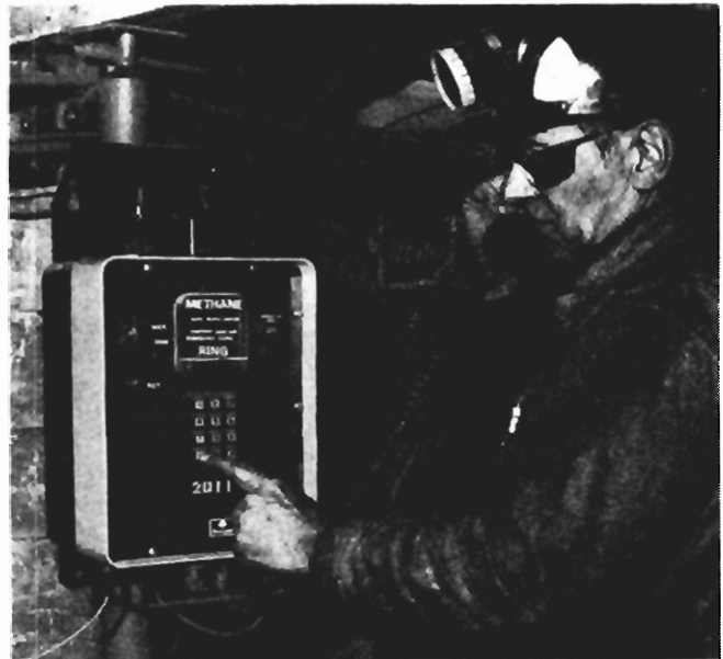
Fig. 44. Underground mine phone using frequency-division multiplex transmission.
