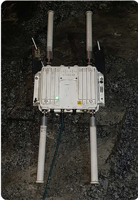
Figure 69 Wall mounted IW3702 within the test Mine
