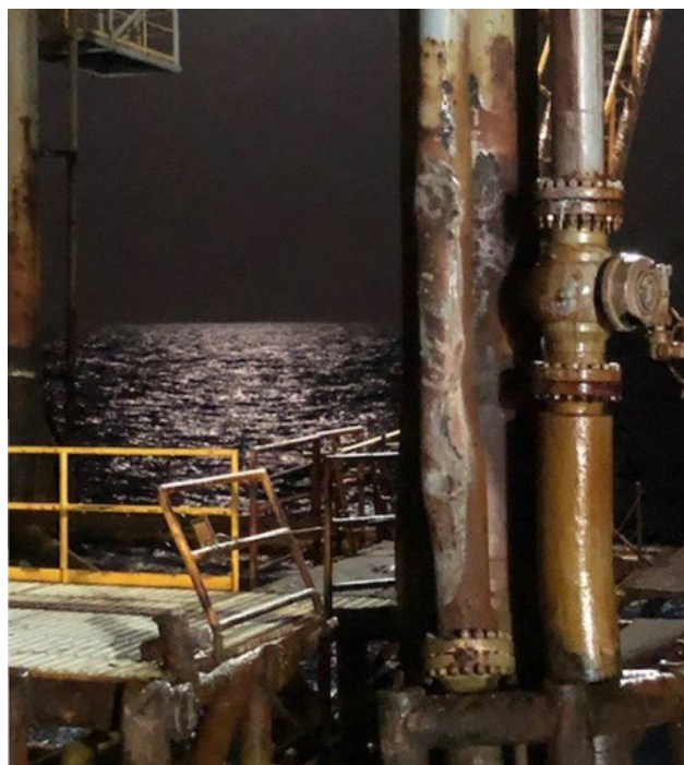
Figure 5. Photo of the damages to EI-259A, taken by a Cox employee around 0500. (Source: Cox Operating)
