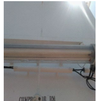
Standing Water in a Certified Safe Flameproof Light Enclosure Indicating Failed Ingress Protection
