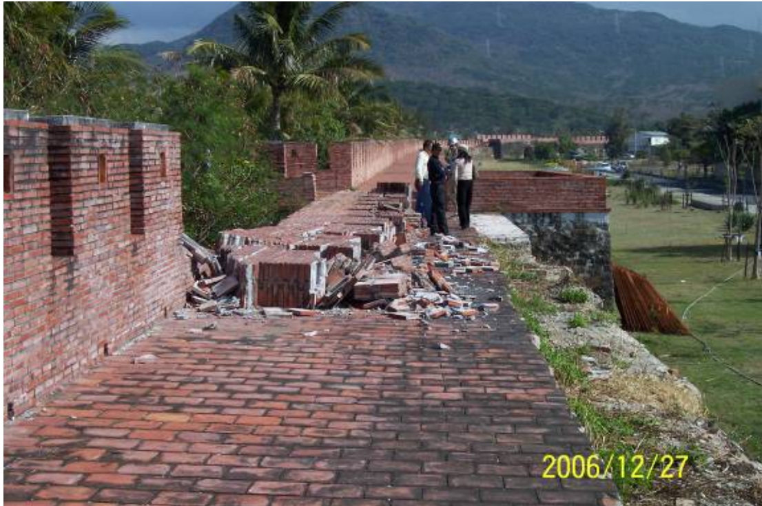
Fig. 16 Battlements of the old city wall at Hengchun were collapsed
