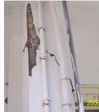
Fig. 14 Shear cracks were due to the short column effect
