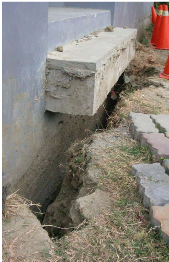
Fig. 22 Ground settlement and lateral displacement observed in school near Nanwan
