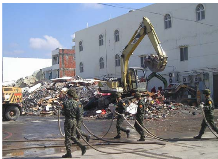
Fig. 9 Front view of the collapsed furniture store
