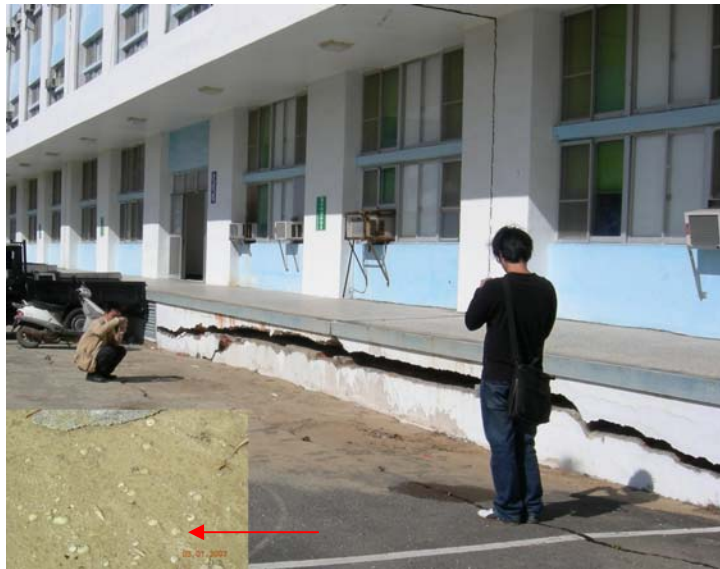
Fig.24 Ground settlement, Soil liquefaction and building damages observed near Nanwan, the shells were found in the sand
