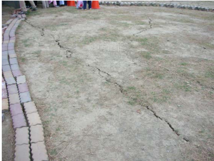
Fig.21 Ground cracks observed in school near Nanwan
