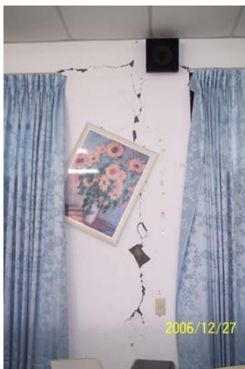
Fig. 13 The damaged column along the direction of the corridor
