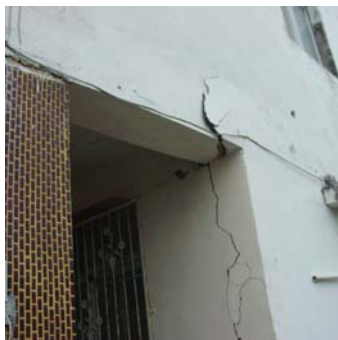
Fig. 12 The damage on the brick walls and beams
