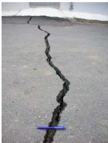
Fig.20 Crack observed near Nanwan
