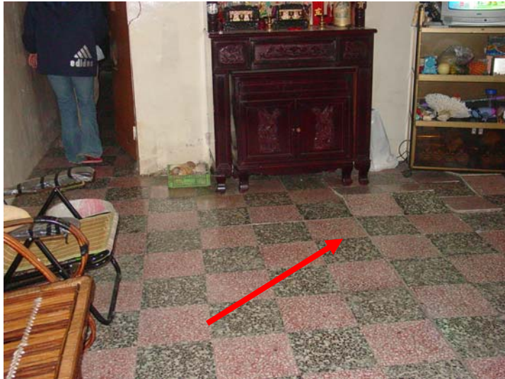
Fig. 11 The ground bulged inside the house
