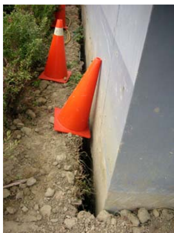
Fig.23 Ground settlement observed in school near Nanwan
