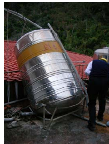
Fig. 15 The collapsed water tank on top of the school building
