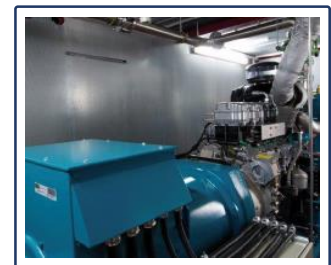
Heat & Power Generation
