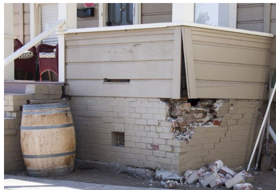
Photo of damage to unreinforced masonry building in South Napa Earthquake.
