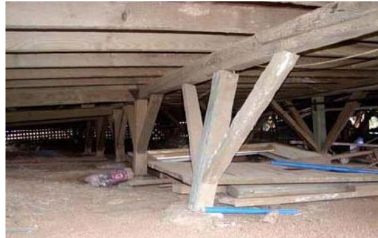
Photo of damage to post and piers in Hawaii Earthquake. COURTESY OF IAN ROBERTSON, AVAILABLE AT WWW.EERI.ORG, LAST ACCESSED 7/7/19
