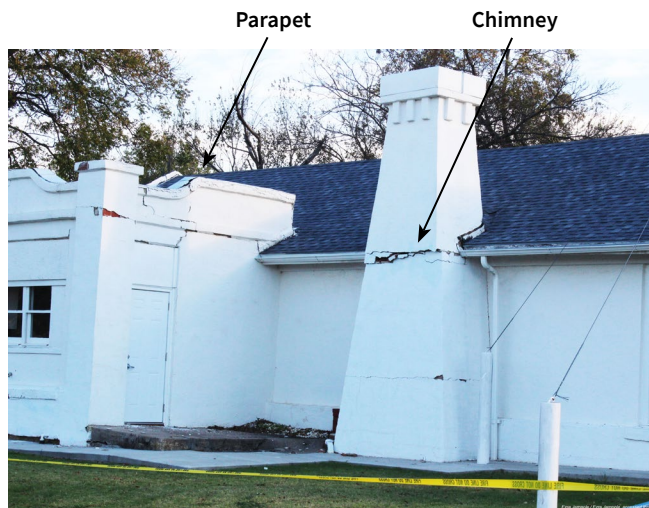
Masonry parapet separation.
