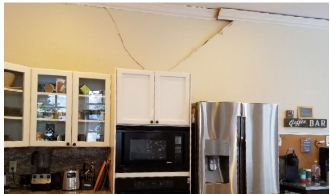
Significant cracking of wall finish materials. PHOTOS OF DAMAGE TO WALL FINISH MATERIALS FROM ANCHORAGE EARTHQUAKE. COURTESY OF JANISE RODGERS, AVAILABLE AT WWW.EERI.ORG, LAST ACCESSED 8/3/19
