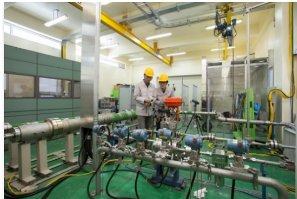
Figure VHTR 6. Small-scale nitrogen gas loop used for studies involving sulphuric acid decomposition and SiC coated process heat exchangers
