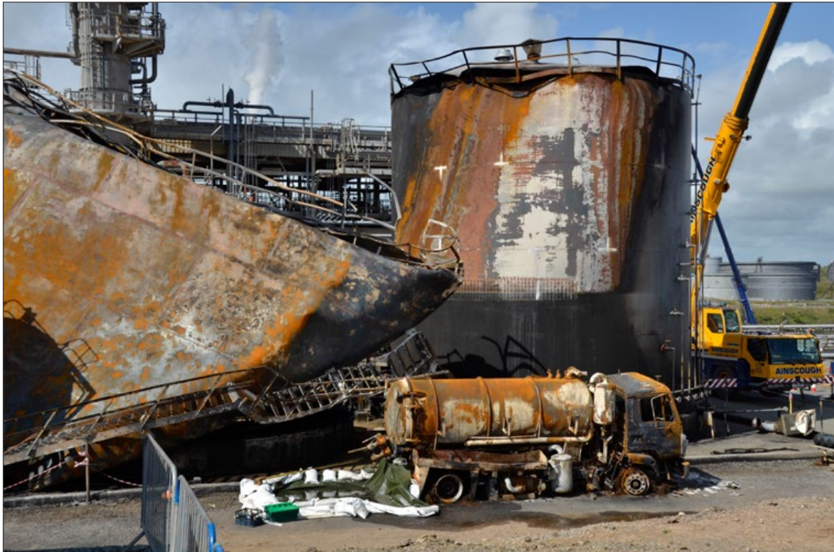
Figure 11 Post-incident – tank 17T302 minus vessel roof
