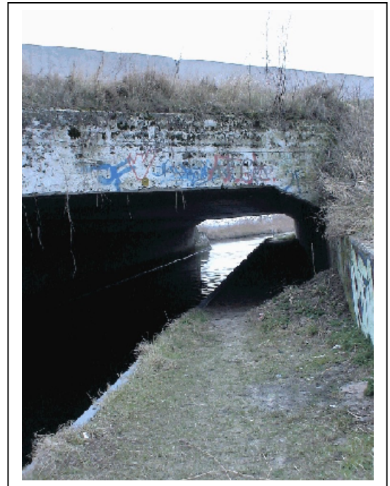
Figure 5 - An adaptation made to an existing water passage under a highway. This lateral ledge was constructed after the road construction.
