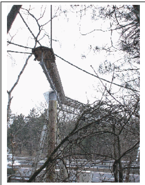
Figure 11 - Adaptation of an information structure over a highway in order to allow squirrel and pine marten to cross to the other side. This is an experience to see if this kind of structures will be used by these species.
