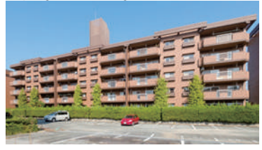
<The fourth building had the largest inclination as pilings were damaged to cause inclination>
