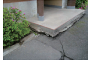
<Subsidence caused liquefaction>
