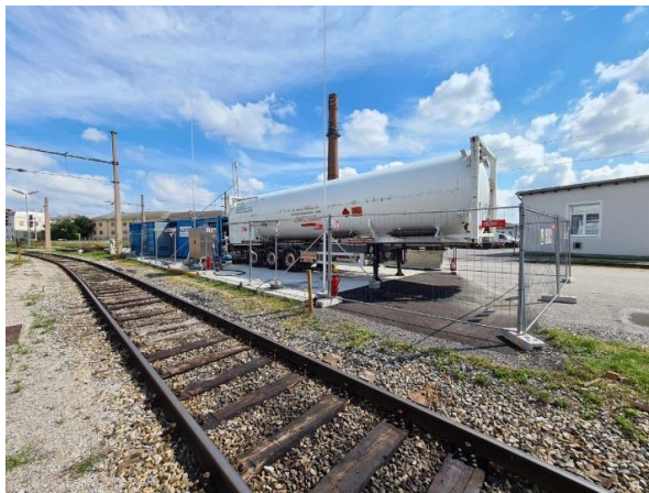
Hydrogen trailer & compressors
