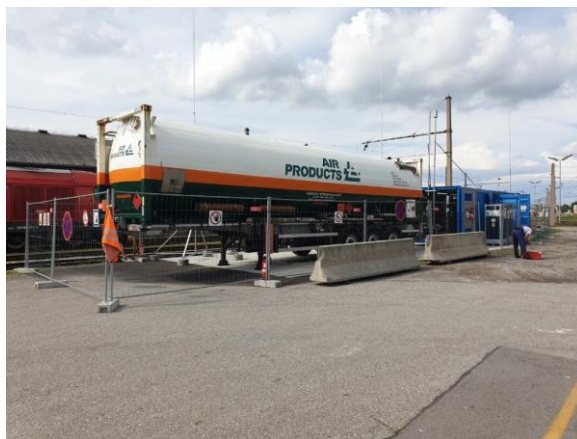
Hydrogen trailer & compressors
