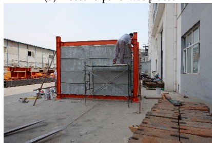
(d) The exposed steel tie bars were welded to the slab of framework columns
