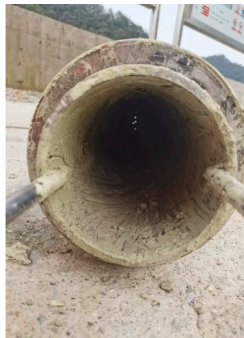
Figure 8. Sulfur deposits in surface pipelines.
