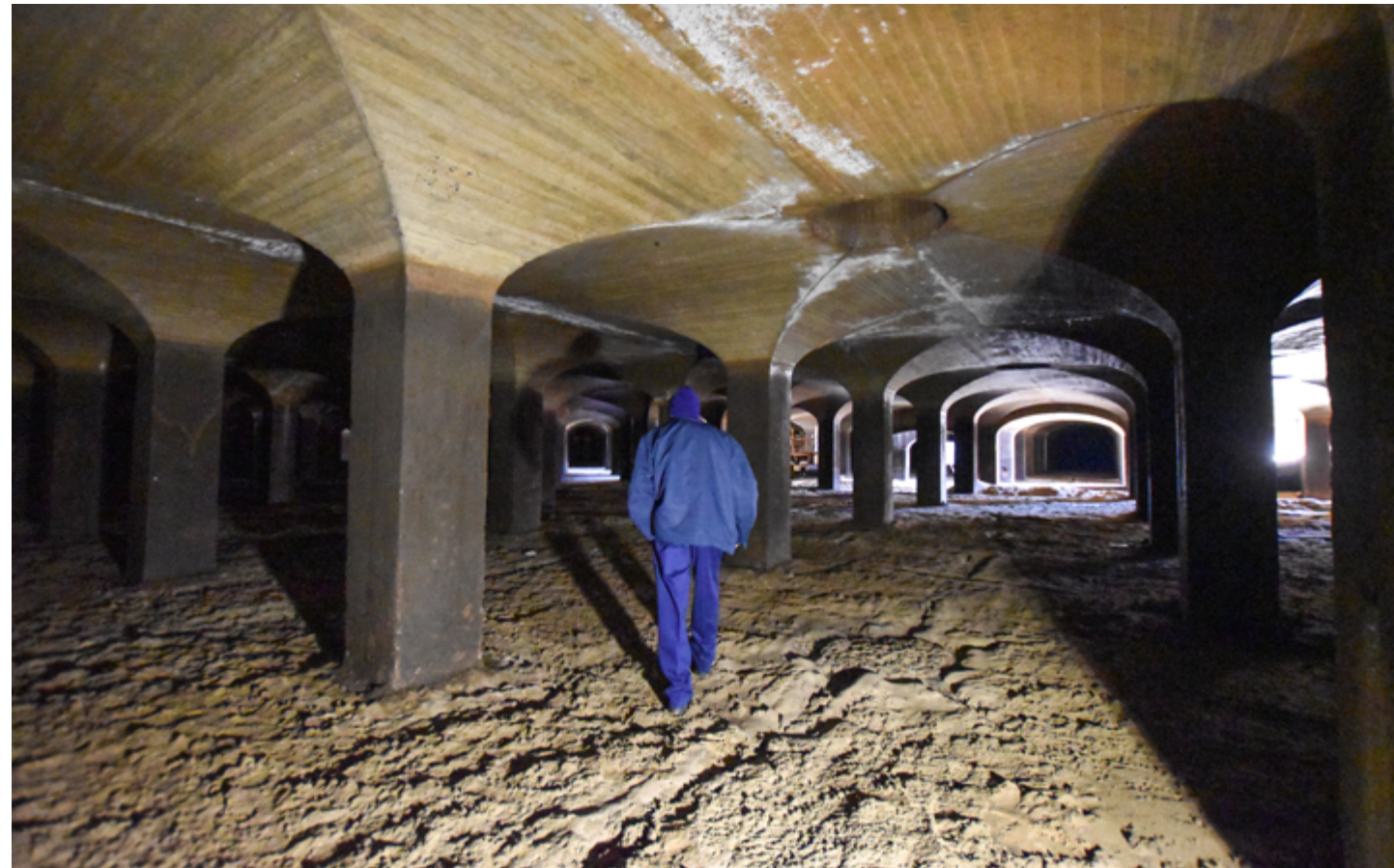
Sand Filter #7, located on the grounds of McMillan Water Treatment Plant in Washington, D.C. (U.S. Army photo by Cynthia Mitchell)
