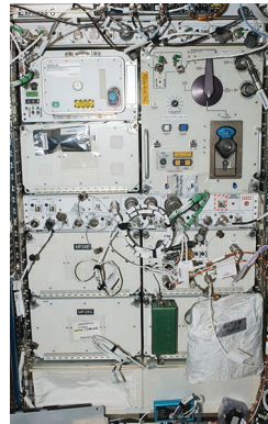
Sub-rack-sized experiments with standard utilities such as power, data, cooling, and gases.
