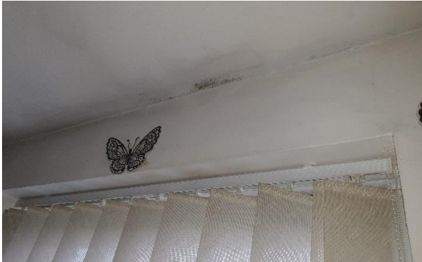
Image 5 - An example of mould inside PRSMANC5's living room
