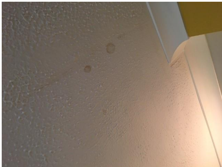
Image 4 - The stain from a recurring leak in PRSWAF11's lounge
