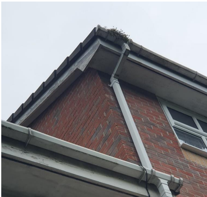
Image 1 - Image 1 - Leaks inside OOMANC2's dwelling were attributed to issues with her gutters
