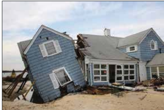
Mantoloking, NJ, January 16, 2013 — Home in this bayside community suffered severe damage after Hurricane Sandy struck the area. FEMA Public Affair / Photo by Adam DuBrowa
