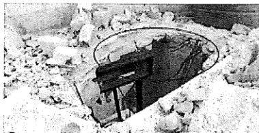
The dimensions of the crater in the roof are 165x106 cm The presence of sticking out rebar elements consisting of soft and loose wires inside the crater indicates that it was widened intentionally in a mechanical way
