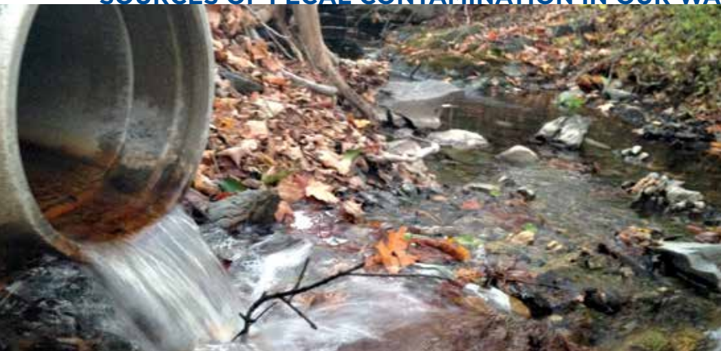
A pipe discharges treated sewage effluent on the Indian Kill, a tributary of the Hudson River. Photo by Dan Shapley/Riverkeeper.
