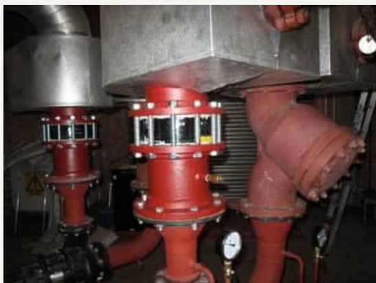
New non return valves were fitted to the existing pump sets to allow smoother integration of the WSHP.
