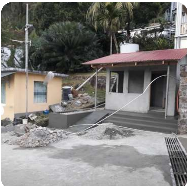
The new Security Guard post during the construction phase (The old one is adjacent)
