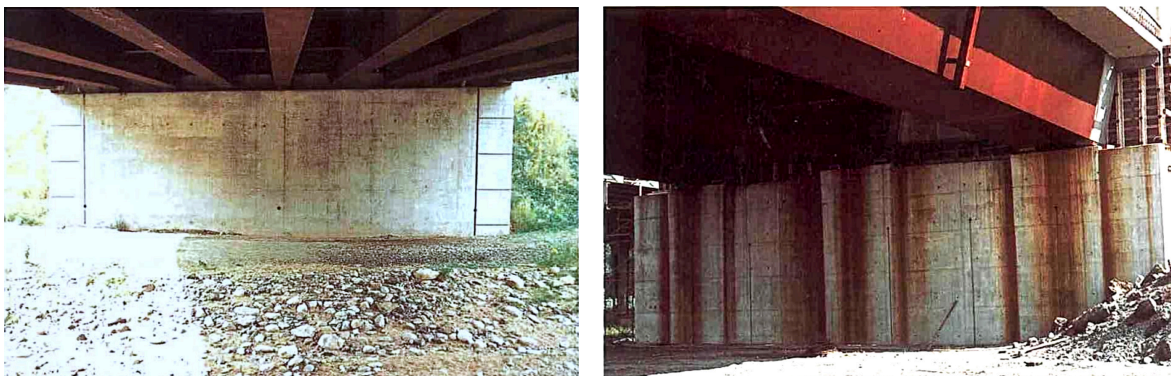
Fig. 3.17: (left) Abutment free of rust as a result of a good detailing and drainage and (right) abutment with severe rust staining due to bad detailing
