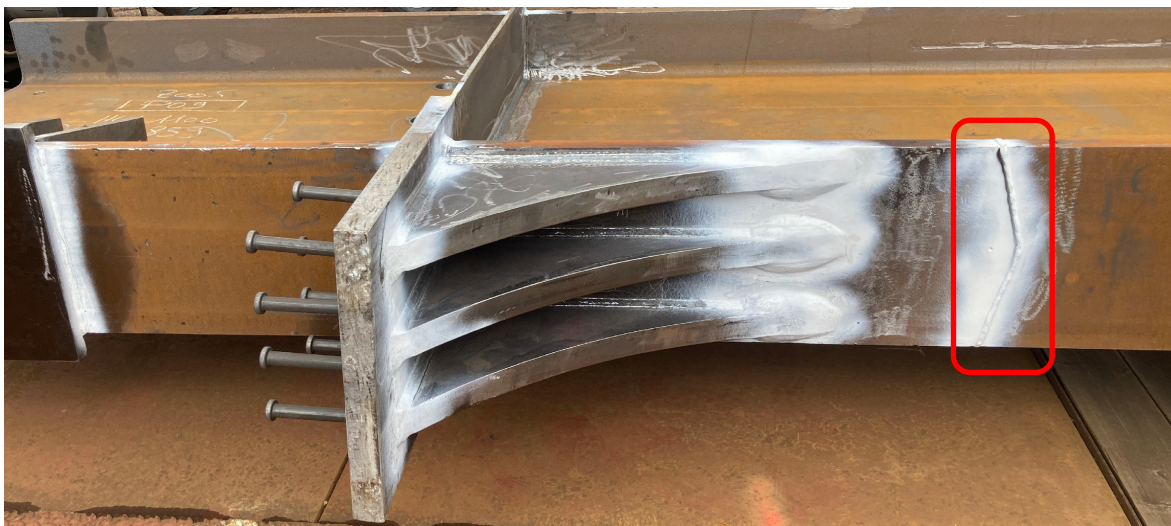
Fig. 3.16: Example of welded seams as drip edges for an integral bridge without expansion joints
