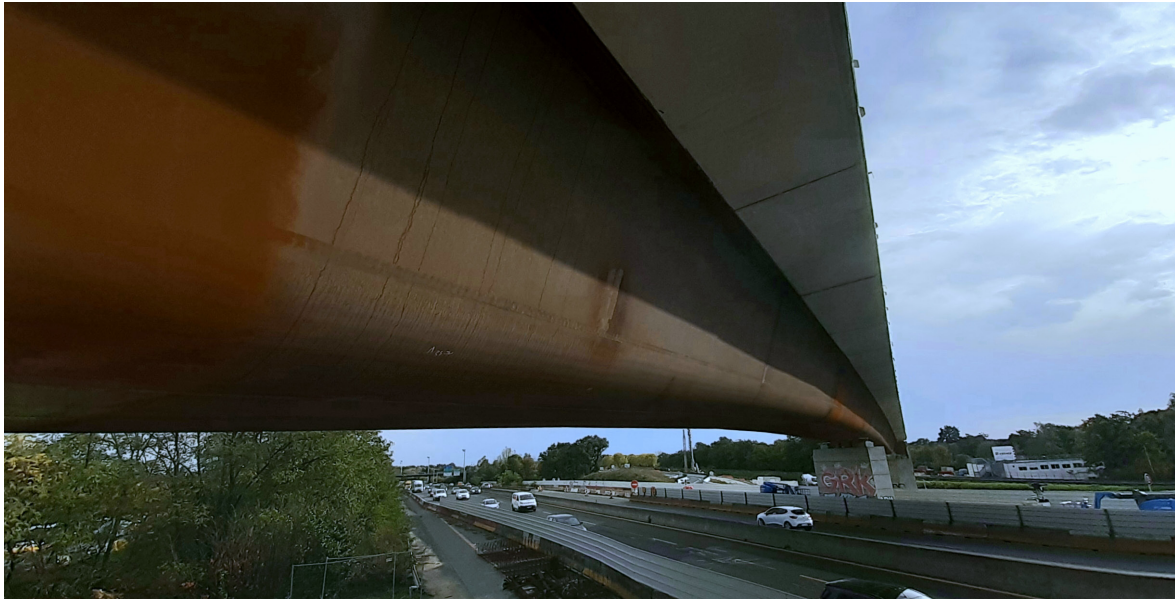
Fig. 2.26: Composite bridge with weathering steel box girder over a highway in Evry-Courcouronnes, France
