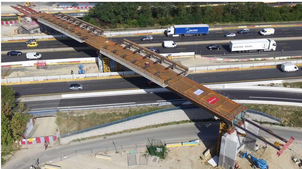
Fig. 2.27: Erection of the box girder for the composite bridge in Evry-Courcouronnes, France, in 2019
