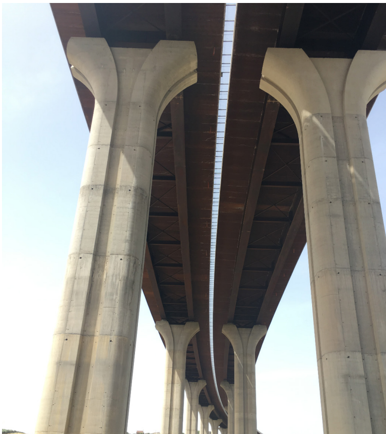
Fig. 2.20: Road viaduct in Sicily (Italy) with decks completely made of weathering steel
