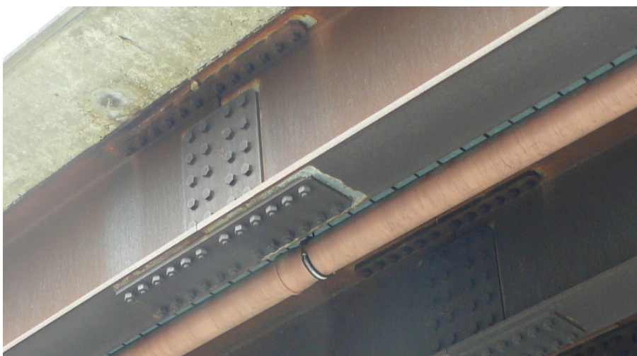
Fig. 3.21: Slip resistant connection with preloaded weathering steel bolts and an alkali-zinc-silicate paint on the contact surfaces at the Howald bridge in Luxembourg
