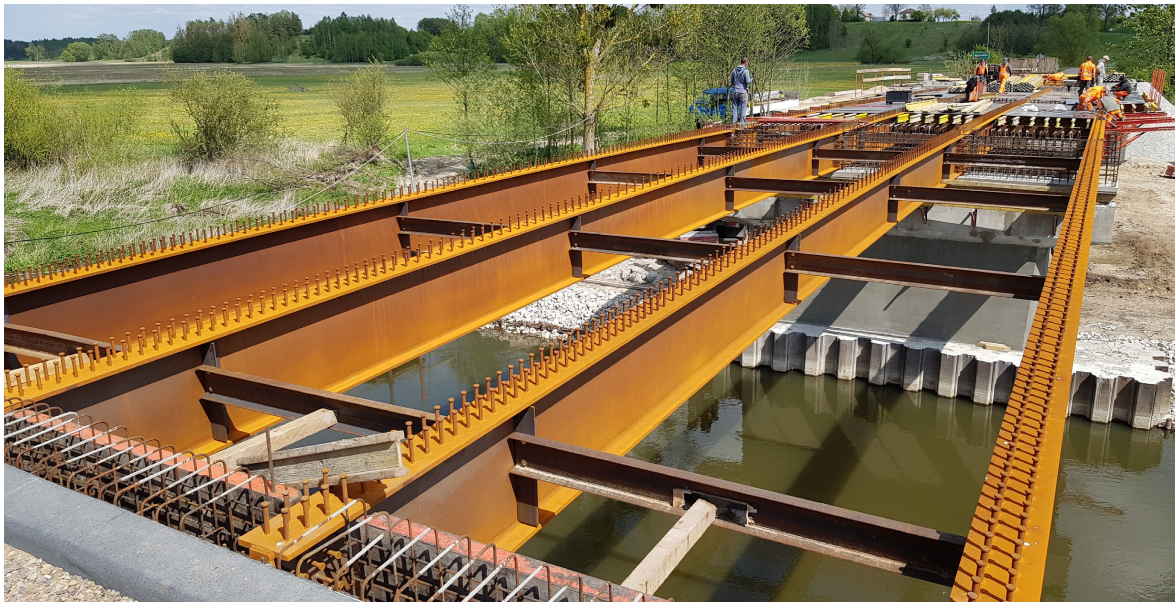
Fig. 2.29: Weathering steel girders at the erection of the composite bridge in Wirkowice (Poland) with a light orange-brown oxide layer after short exposure for several weeks
