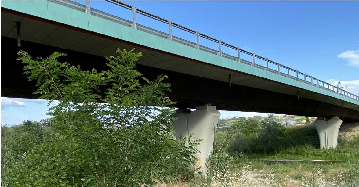
Fig. 2.21: Composite bridge with box girder over the Cesano River in Marche Region, Italy
