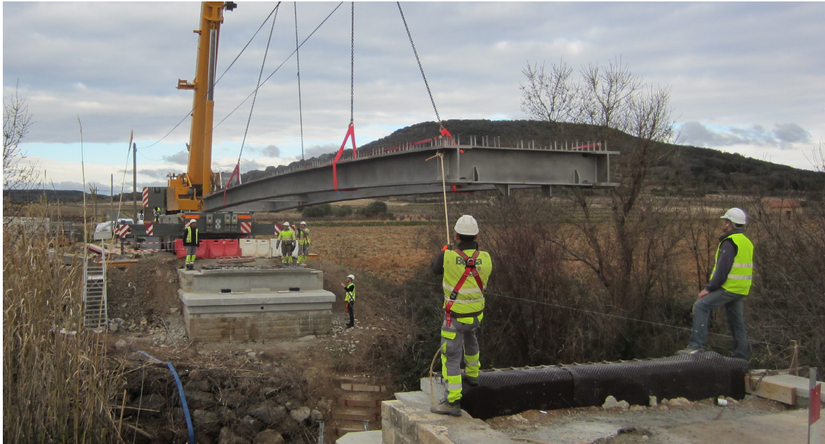
Fig. 2.5: Composite bridge during assembly of steel structure without oxide layer, San Martin à Fontes, France
