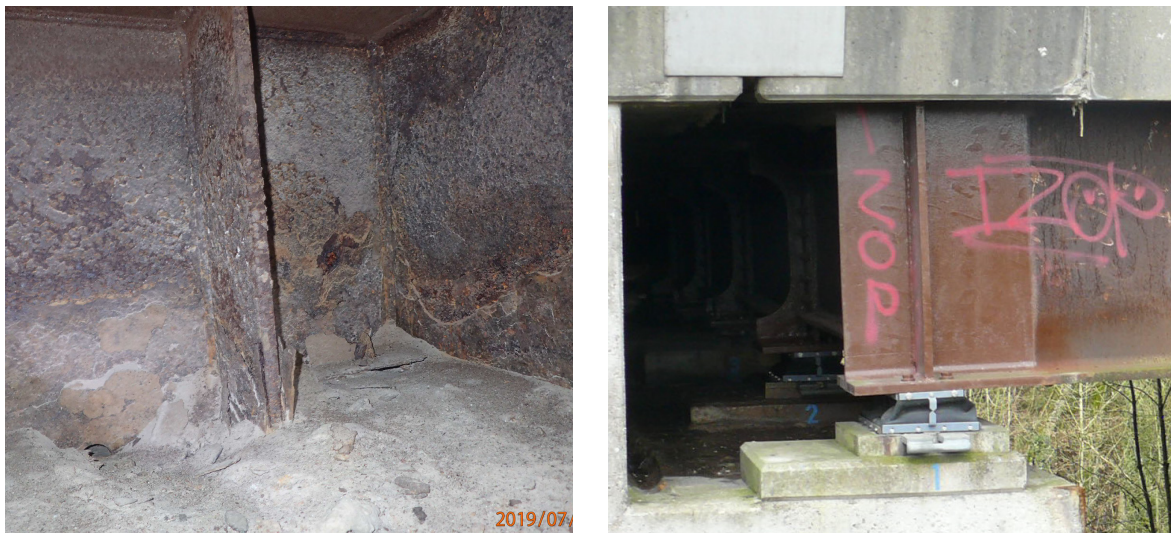
Fig. 3.11: (left) damaged oxide layer because of a leaking expansion joint and bad drainage system at the abutment and (right) a local rehabilitation of a damaged area with a subsequent corrosion protection paint
