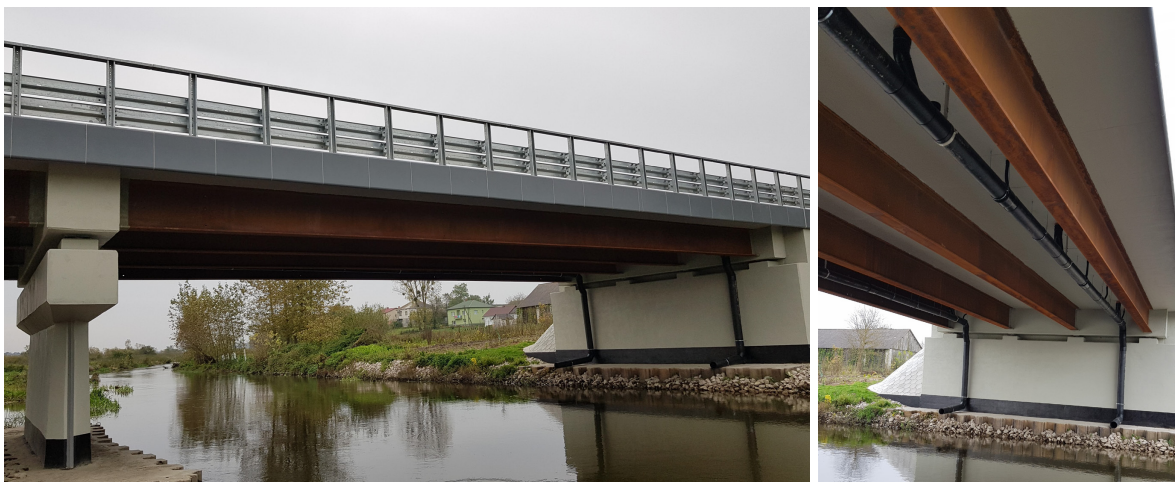
Fig. 2.30: Completed composite bridge over the Wieprz River in Wirkowice (Poland) with an orange-brown oxide layer after exposure for six months
