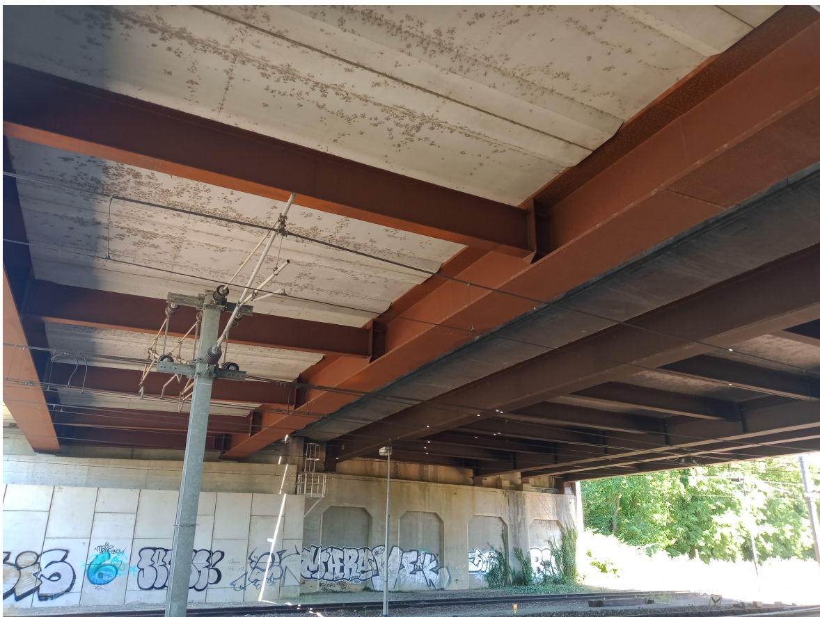
Fig. 2.28: Saumur bridges in Saumur, France, build in 2015 (new bridge on the left) and 1982 (two bridges on the right)
