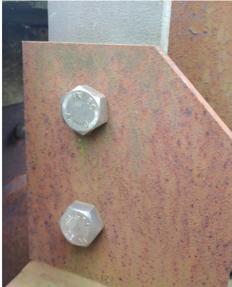
Fig. 3.23: A4 stainless steel bolts at a footbridge made of weathering steel after 12 years in service
