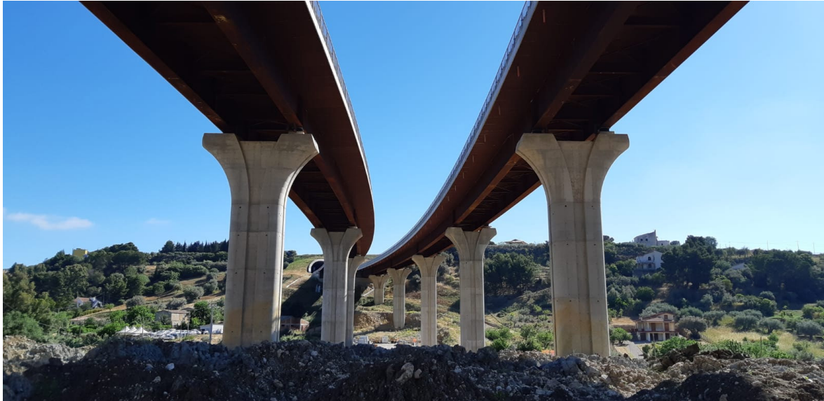
Fig. 2.19: Road viaduct in Sicily (Italy) with decks completely made of weathering steel
