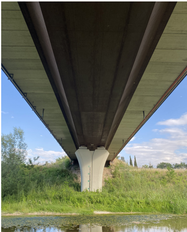
Fig. 2.22: Composite bridge with box girder over the Cesano River in Marche Region, Italy
