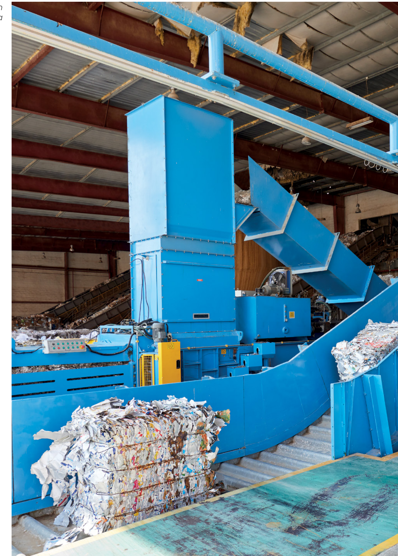
Recycling facility in Saudi Arabia
