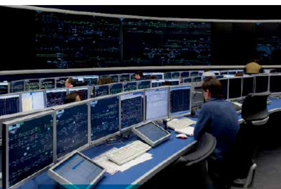
Rail traffic control centre
