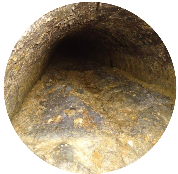
FOG blocking our sewer pipes which can lead to flooding and pollution to homes, businesses and the environment.
