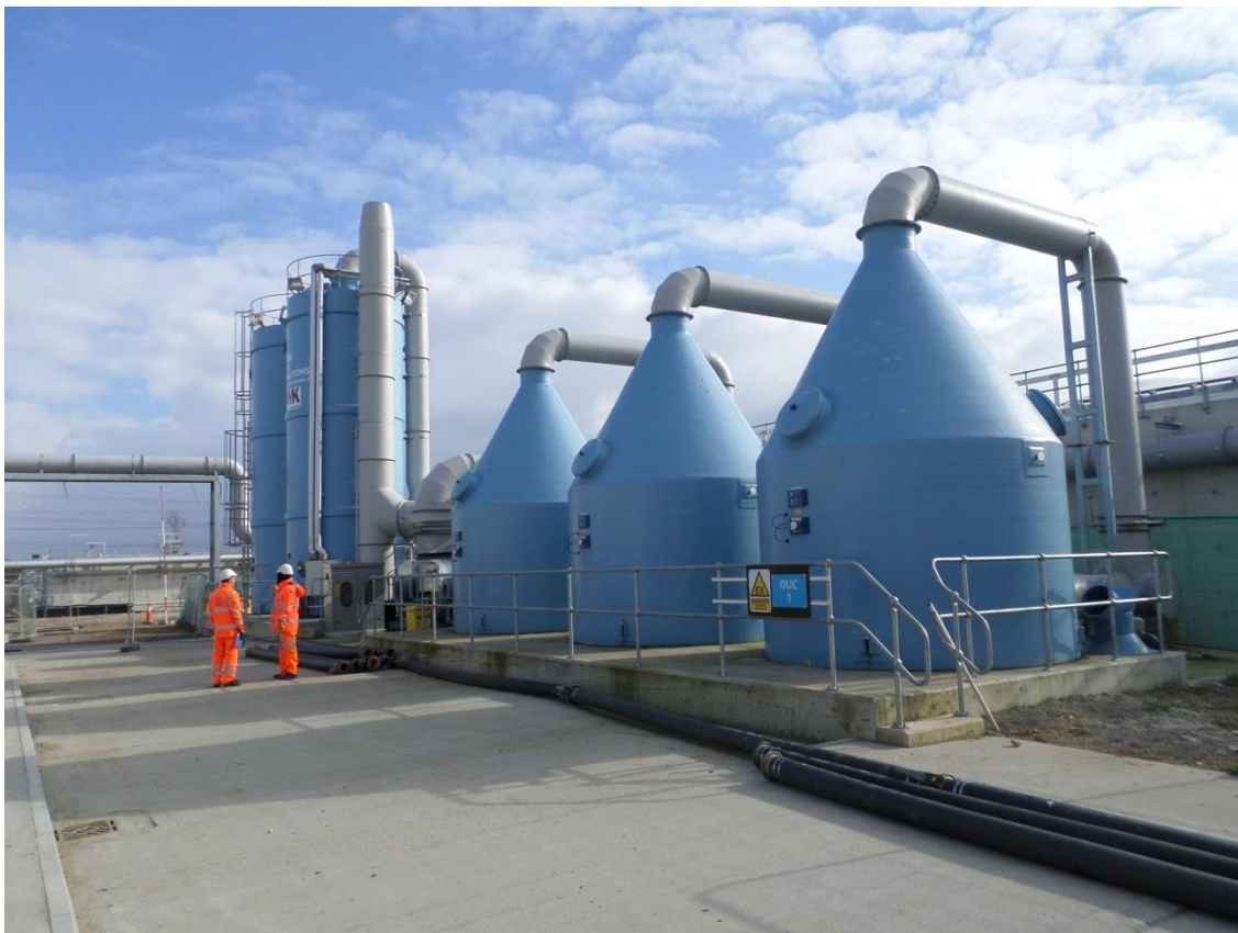
An odour control unit at Deephams sewage treatment works.
