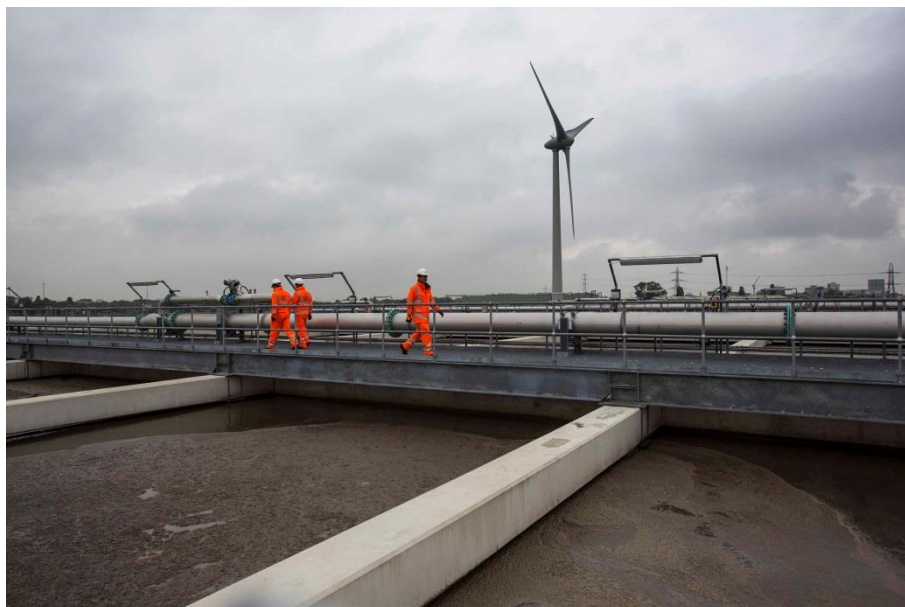
Aeration lanes at Beckton sewage treatment works.
