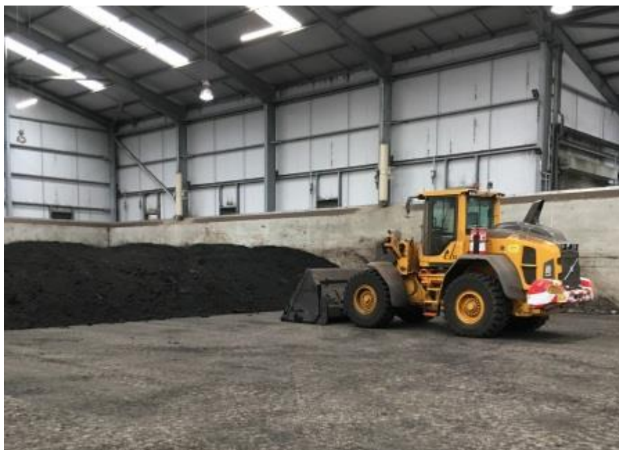
Sludge cake storage at Long Reach sewage treatment works.
