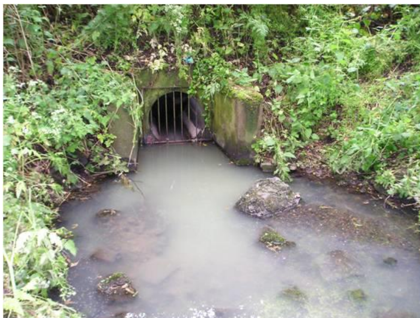
A polluted outfall, before misconnection investigations have been carried out.
