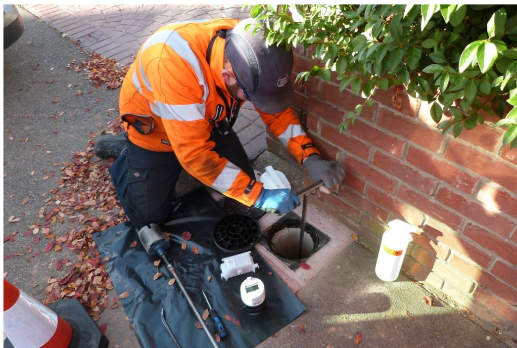
Installing a smart meter at a customer's home.
