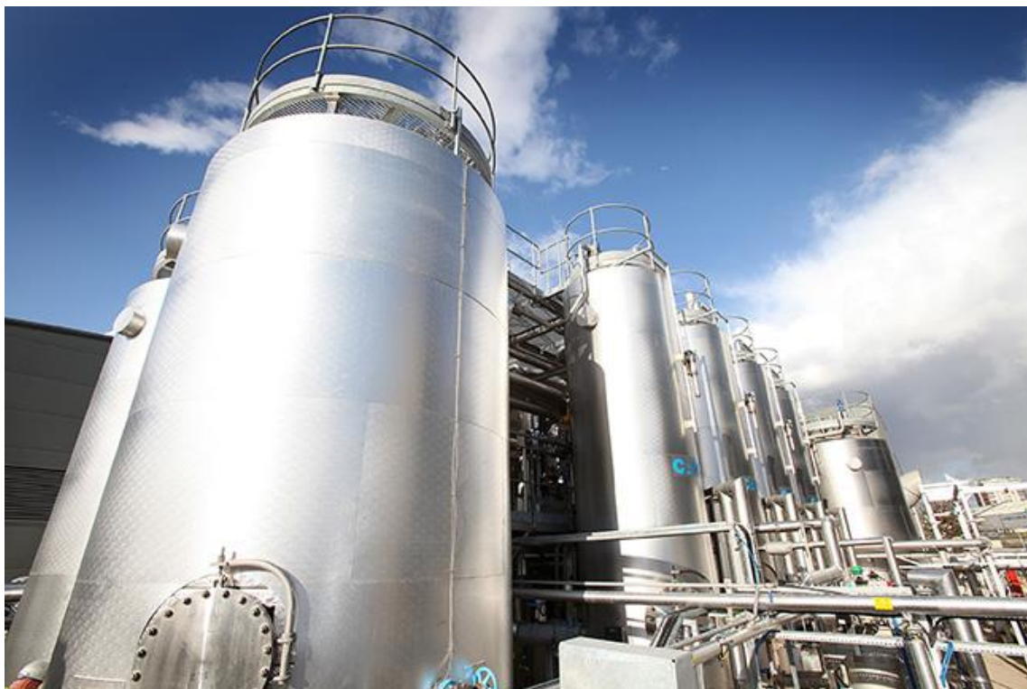
Thermal Hydrolysis Plant (THP) at Riverside sewage treatment works.
