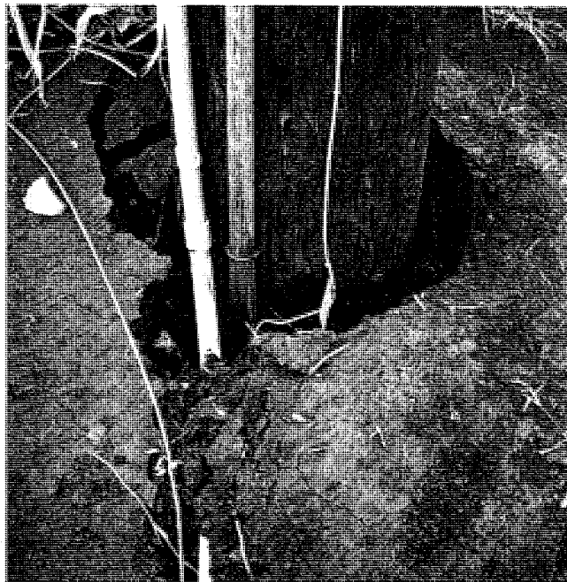
Hanapepe LARC site showing the force of Hurricane Iniki's winds. The pole moved a total of 8 inches; the gap at the base measured 4 inches.
