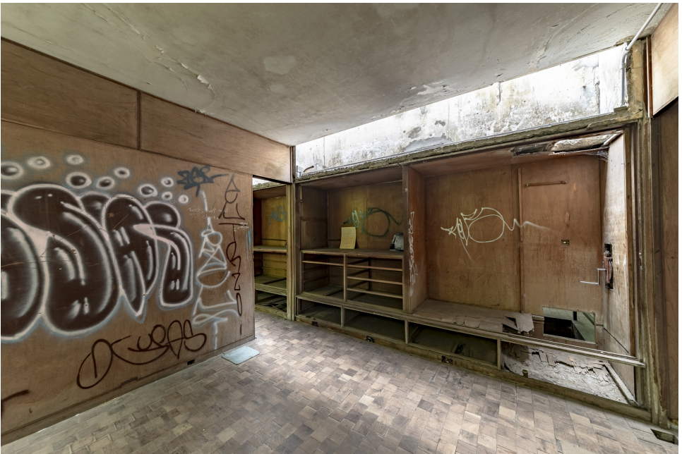
Graffiti and other damage to the interiors of the Casa sobre el Arroyo before restoration.
