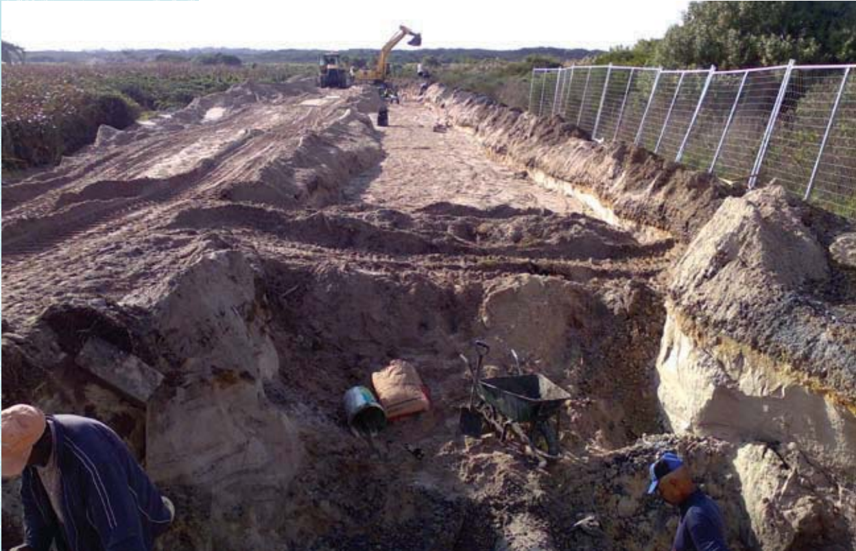
Construction of the “cut-off canal” to protect Zeekoevlei from seepage from the Cape Flats WWT works. (Photo: Candice Haskins)
