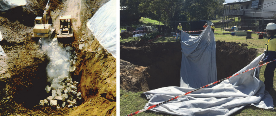
Figure 6. Bulldozing chunk rock into the throat of a large subsidence sinkhole, from [17] (left); installation of the geotextile to line the base and walls of the sinkhole, from [18] (right)
