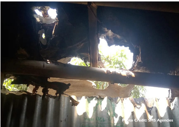
Image: Partially Damaged Shelter in Camp 10
