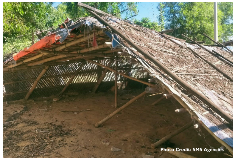
Image: Fully Damaged Shelter in Camp 3
