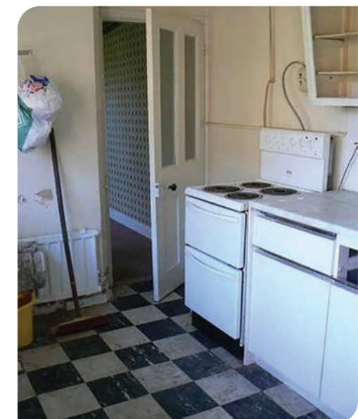
Photo: Flames, hot surfaces hazard as cooker too close to doorway
