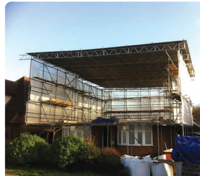
Photo: A modest bungalow in the process of being transformed into a large, two-storey house
