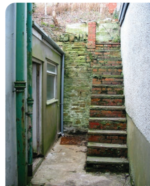
Photo: Falls on stairs and steps hazard
