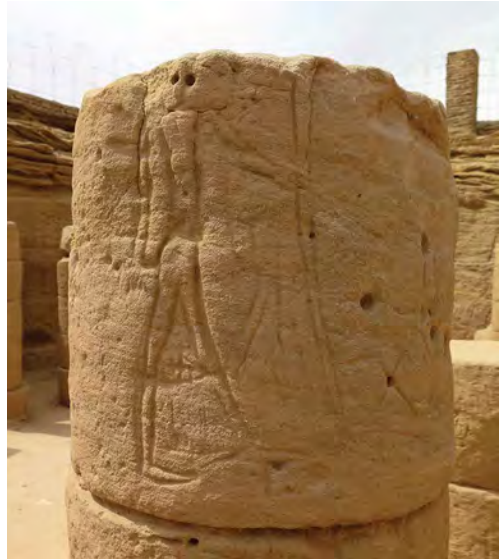
FIGURE 4.3. This important graffiti depicting archers was at high risk due to cracking. Graffiti T1.
