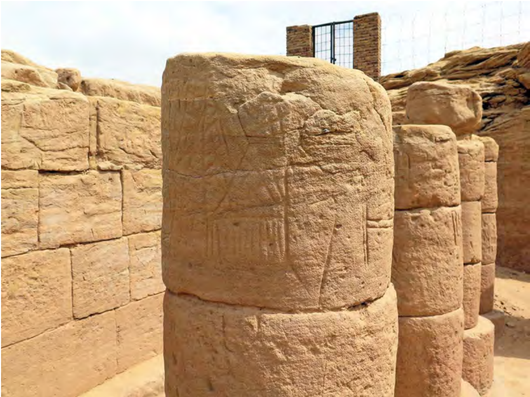
FIGURE 4.1. A column in the El-Kurru funerary temple, showing sanding, cracking, and scaling.
