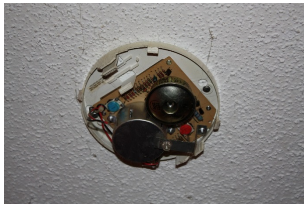
Photograph 2: Uncovered smoke detector wiring.
