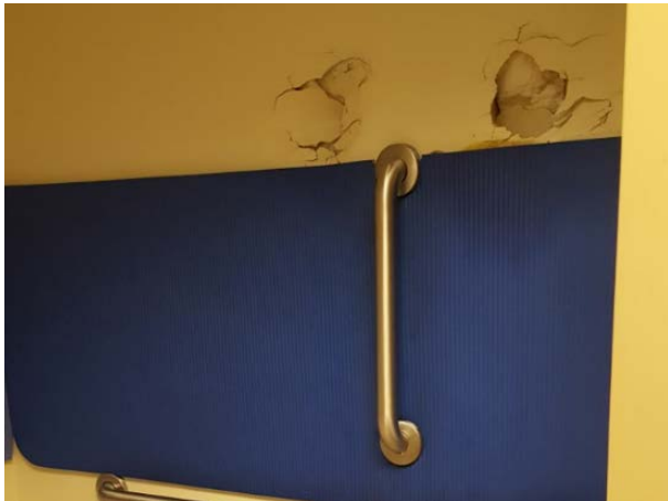
Photograph 1: A wall in a bathroom had holes.
