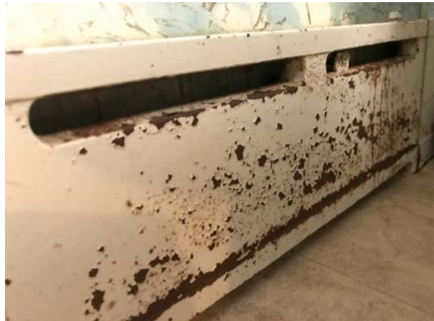
Photograph 2: Rust covered a bathroom radiator.
