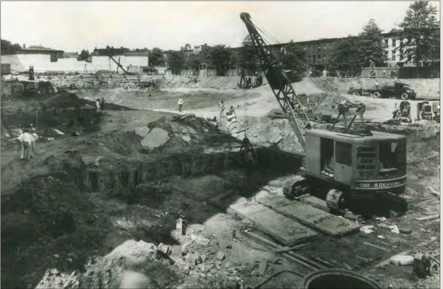
Excavation of the basement of Building 3. The row houses on H Street NW stretch across the upper part of the photo.
