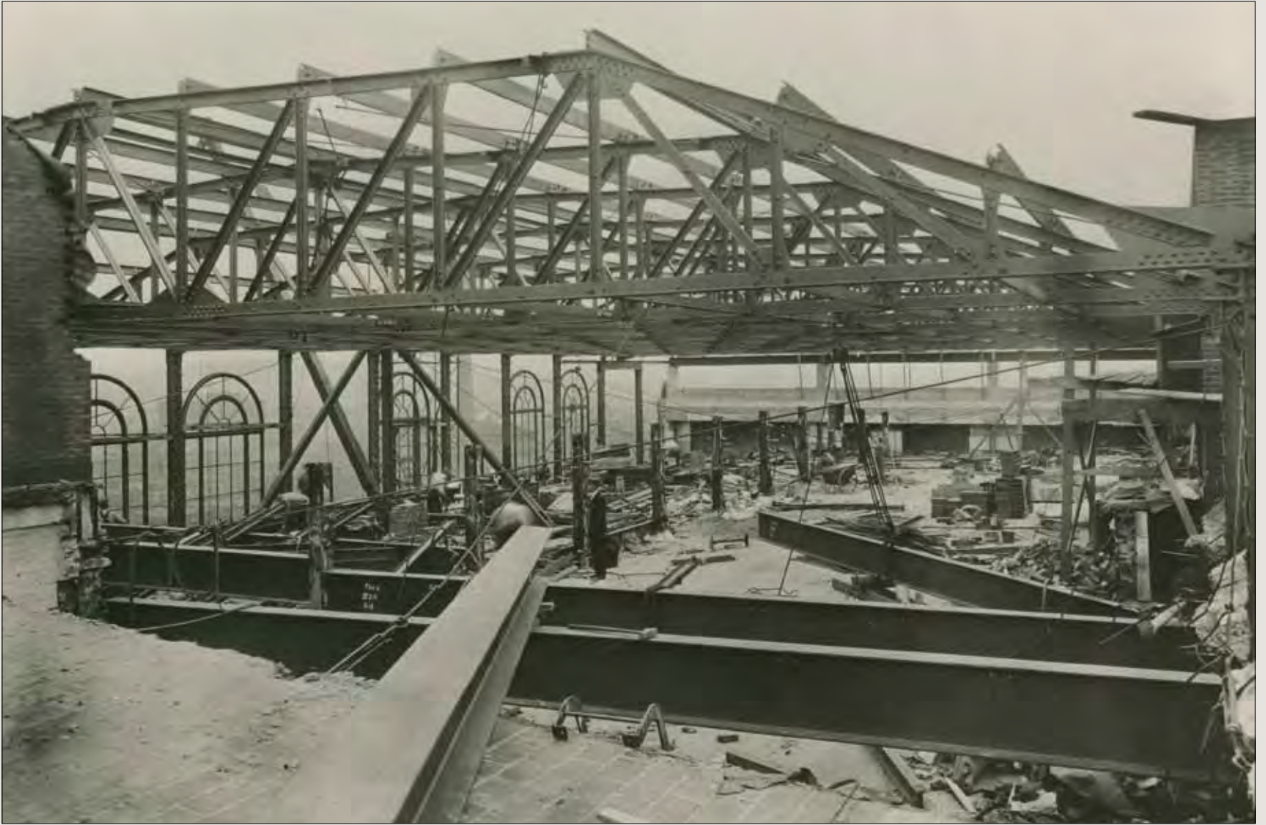
In 1929, an enlargement of Harding Hall was authorized. The roof was raised, a balcony was added, and the new hall seated 1,800. It was dedicated in May 1930.
