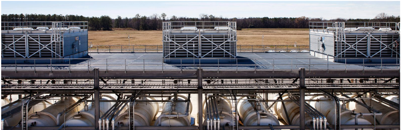
Onsite water storage tanks and cooling towers at our data center in Berkeley County, SC
