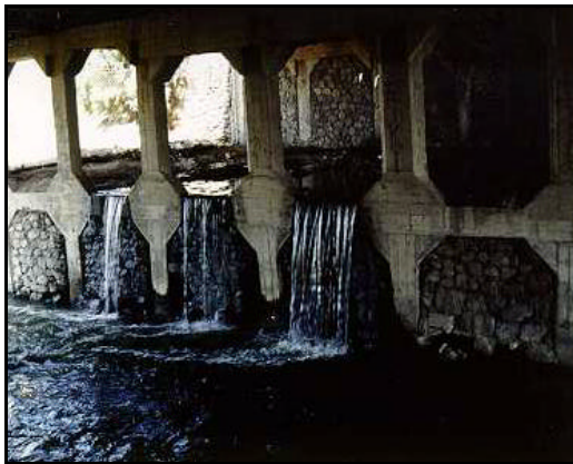
Figure 142: Bypass of raw sewage at Av. Reforma crossing from east bank (Aug 1994)
