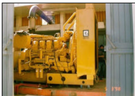
Figure 196 - Standby generator at Pumping Plant No. 1 (Mar 1998)
