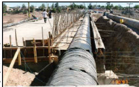
Figure 188: Replacement of concrete pipe with steel pipe on the South Collector (Jan 1997)
