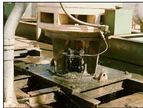
Figure 109: Worn out pump motor at Pumping Plant No. 1 (Nov 1990)
