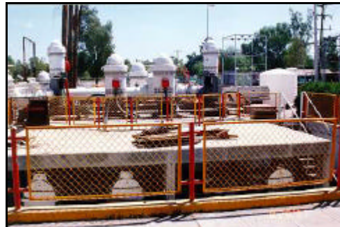
Figure 191: Pumping Plant No. 1 (Aug 1997)
