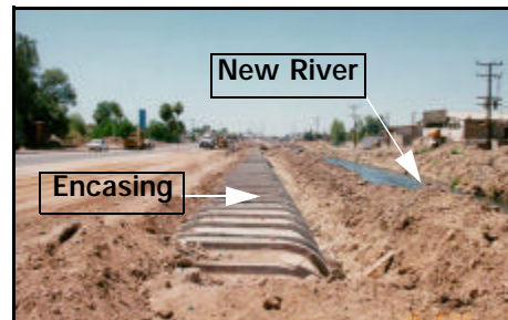
Figure 209 - New River by Pumping Plant No. 2 (Jun 1998)
