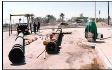
Figure 176: Work underway to correct problems at Pumping Plant No. 3 (formerly PP1A) (Aug 1995)
