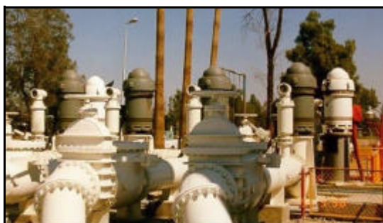
Figure 202 - Pumping Plant No. 1. The new pumps are shown in gray color (Jan 1998)
