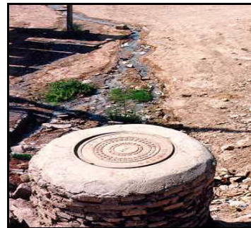
Figure 91: Overflowing sewer manhole (Apr 1988)
