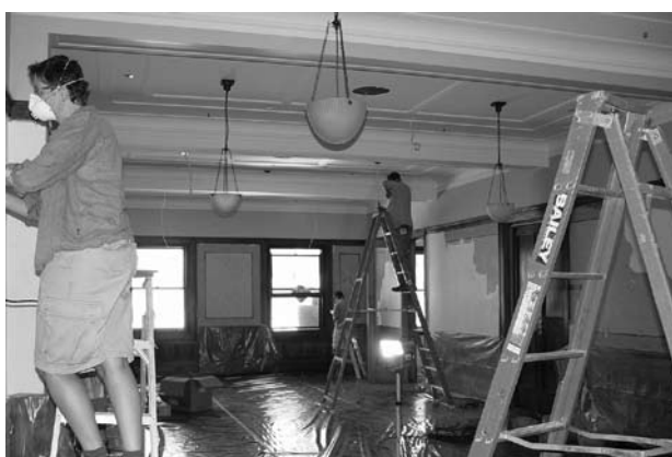
Conservators working on the hand painted wall features in the Members' Private Dining Room
