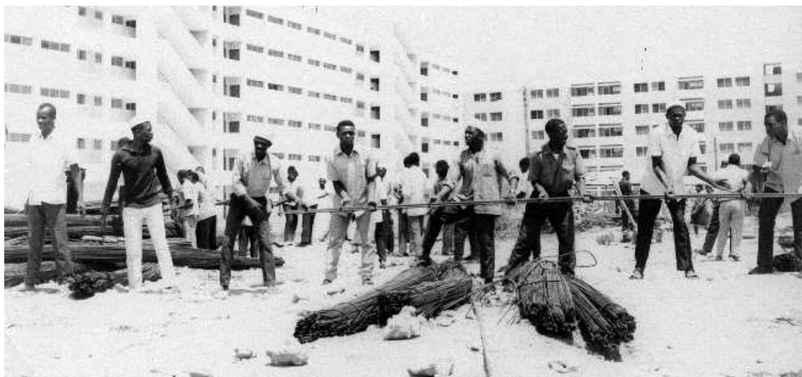
The Michenzani apartment blocks under construction in Stonetown, built with the assistance of the East Germany, and pejoratively referred to as "East Berlin."
