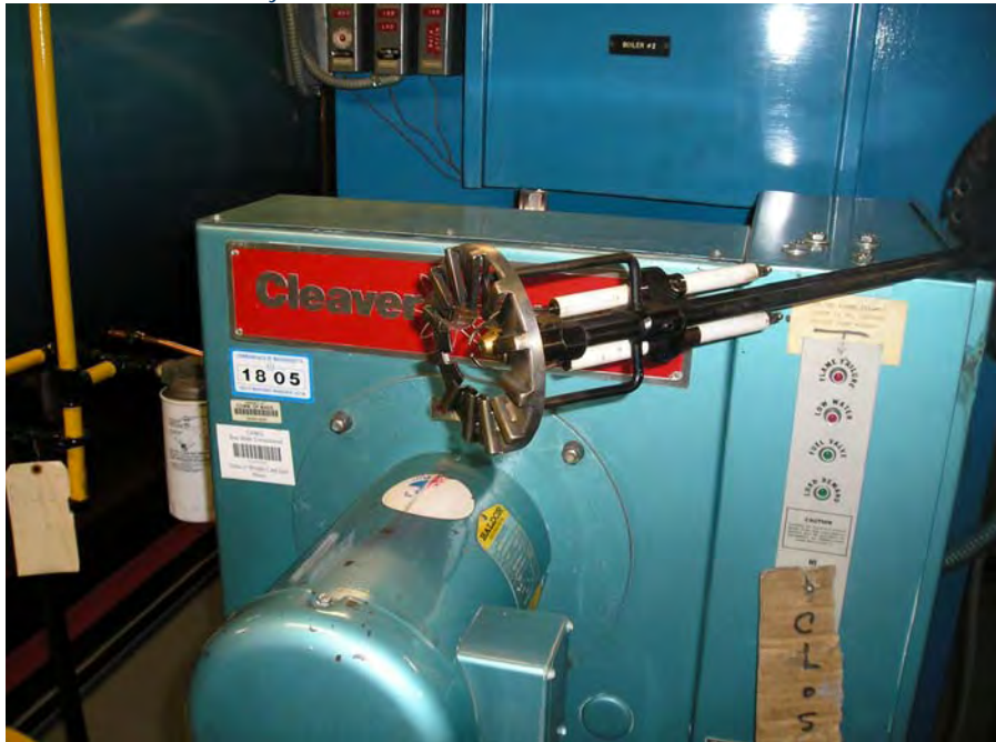
Nozzle Ladder Dirty
