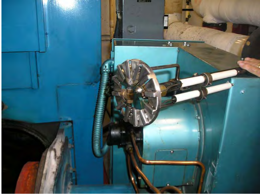
Nozzle Ladder Clean
