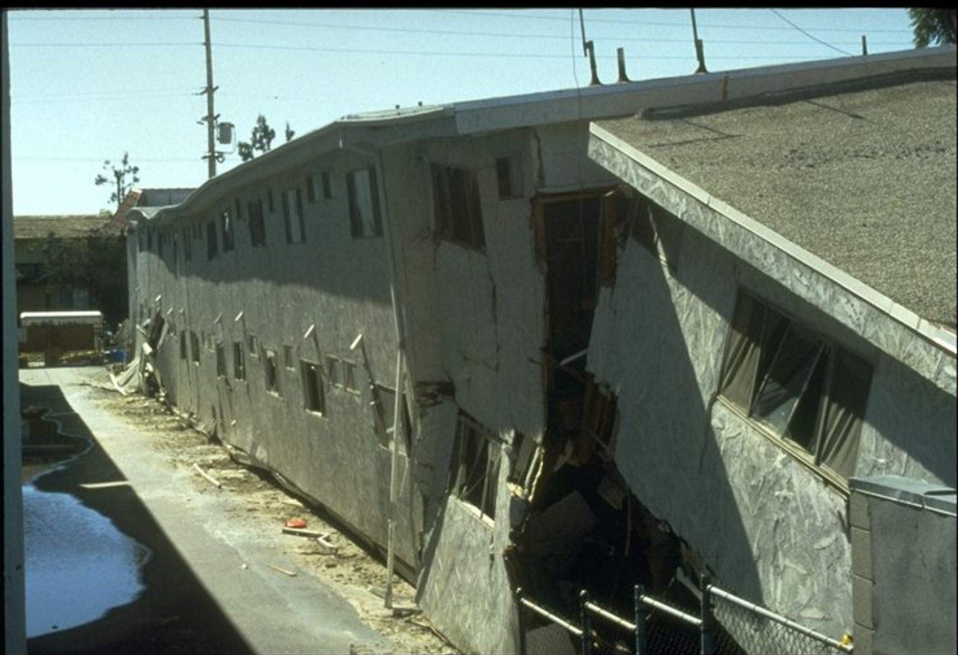
Expect damage to older buildings with soft-story construction (Northridge, 1994).
