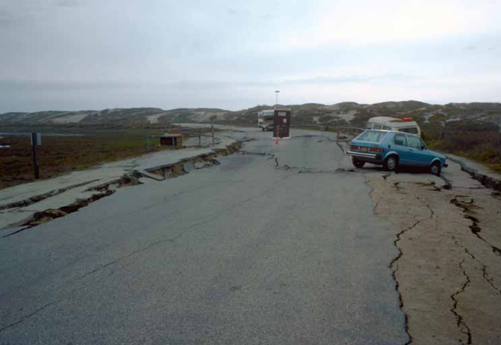
Expect liquefaction (Loma Prieta, 1989).
